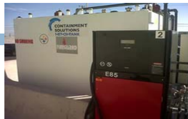
LV Motor Pool Ethanol Tank
